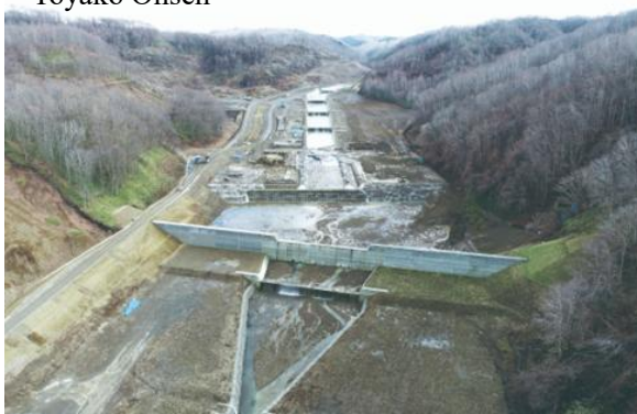
Sabo facilities after earthquake (Hidaka-Horonai River)
